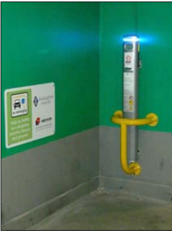
Wall mounted Elektrobay with barrier
